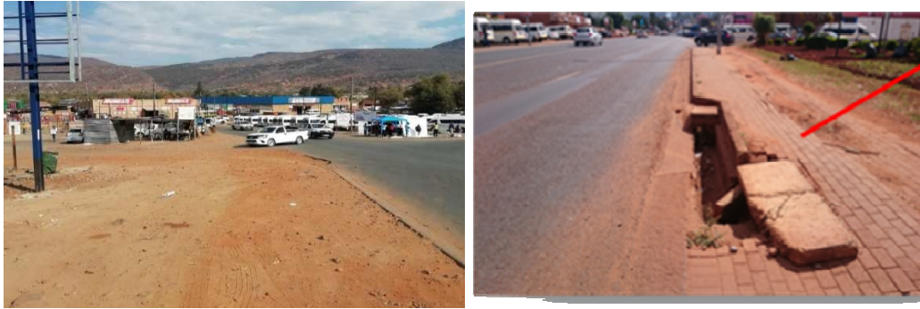
Plate 2: Road and storm water drainage challenges; Source: field work, 2019
