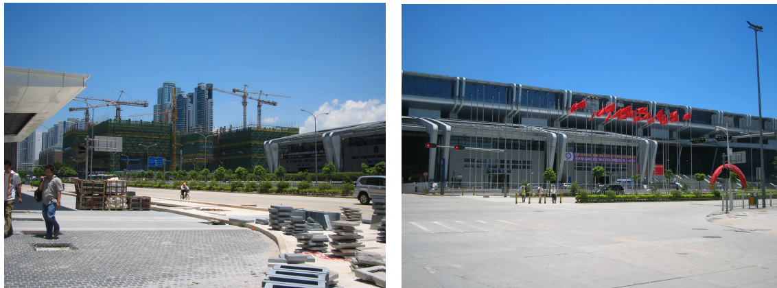
Fig. 5: Shenzhen city convention and exhibition center and other nearby projects under construction. (Photo by author on Jul. 20, 2008)
